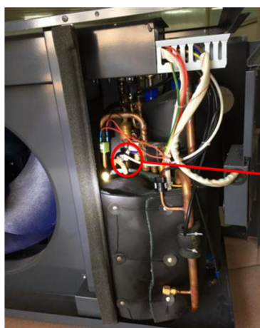
Gas exhaust temp sensor
